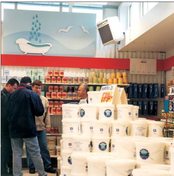
Panther is delivered with adjustable wall mounting brackets which make it possible to direct the air flow for optimal effect and comfort.
